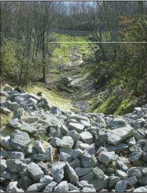
Bear Rock Road in the Crab Creek community has been repaired after being damaged due to a landslide back in 2004. (MIKE DIRKS/TIMES-NEWS)
